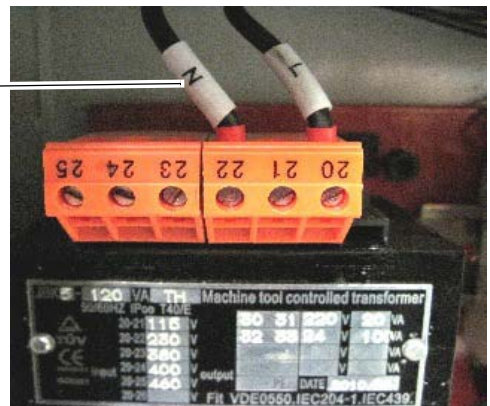
Illustr. 3-6: Transformer wiring
